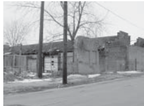
Deteriorated industrial property on East 91st Street
