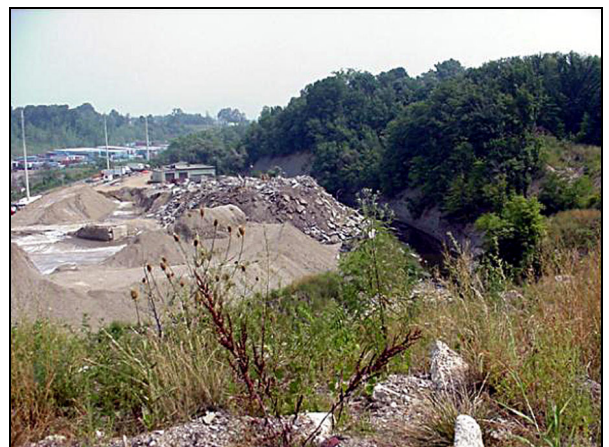
Storage of Construction Material Adjacent to Stream
