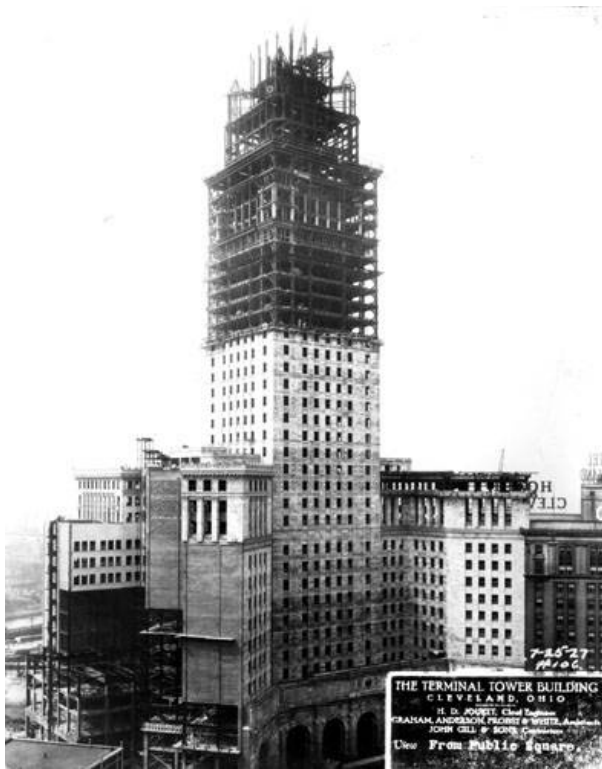
The Cleveland Union Terminal, which was the tallest building outside of New York City when it was completed in 1930, was a ground-breaking development that included commercial retail, hotel, offices, and a railway station.
