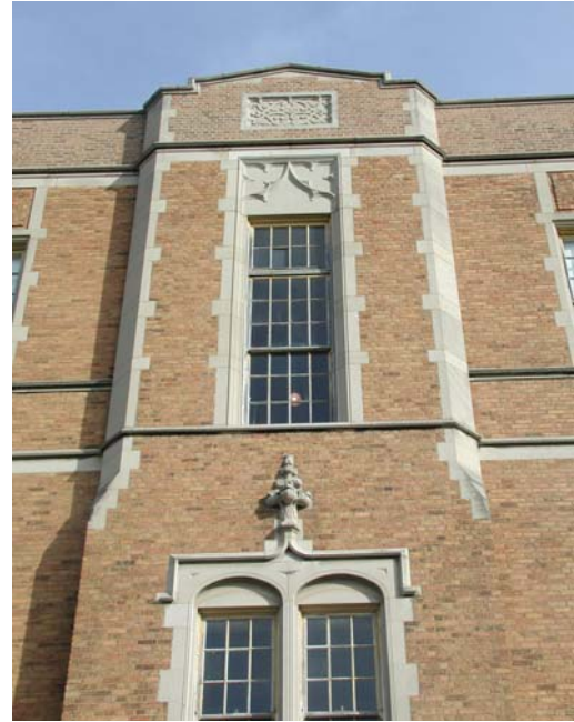
Sandstone details accent window openings and corners on William Cullen Bryant Elementary School, built in 1930.
